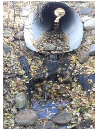
Photo 8: Crossing 2 culvert outlet showing gap that is blocking fish passage and requires replacement.
