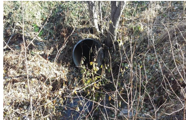
Photo 10: Crossing 2 culvert inlet (under sized).
